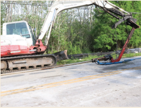
The excavator that came into contact with the overhead powerlines.
